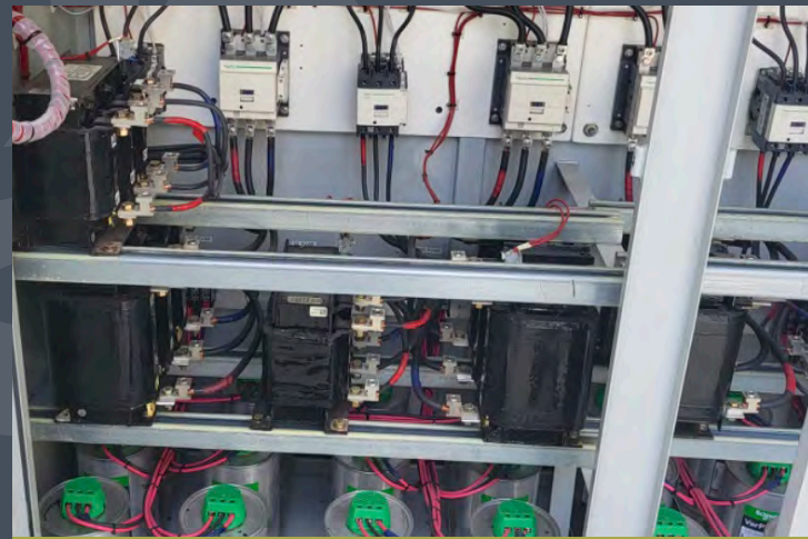
Custom solutions to enhance your electrical usage
