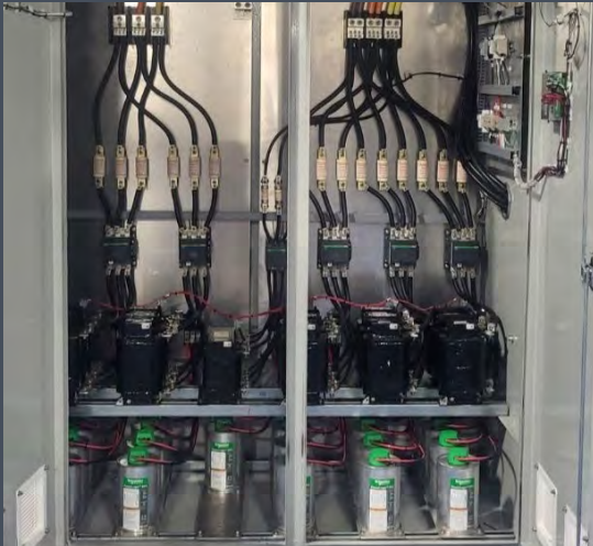
Power Factor Correction opened cabinet
